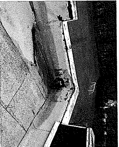
Perimeter condition is falling
